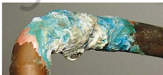
fig-18: Corrosion of copper
